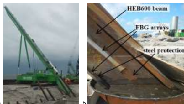
Figure 6. (a) MV pile driving. (b) Installed MV pile with indication of the FBG arrays and their steel protection.
